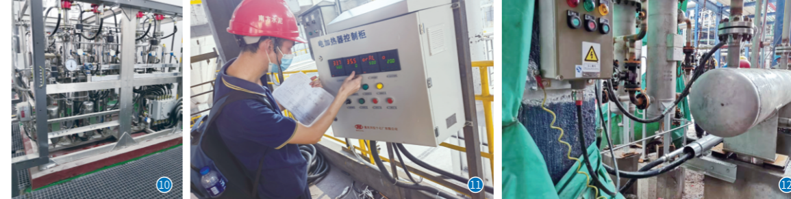
7 COT裂解炉炉管表面热电偶 COT Surface TC
